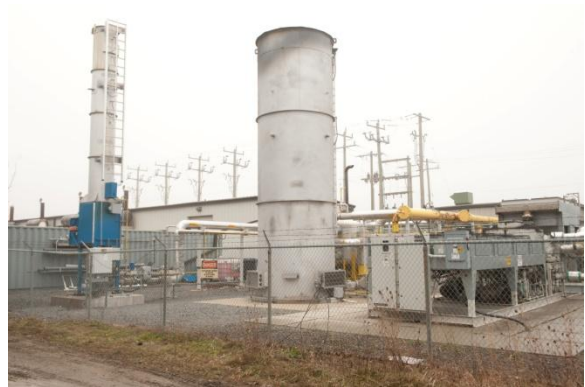
LFG plant at Trail Waste Facility
