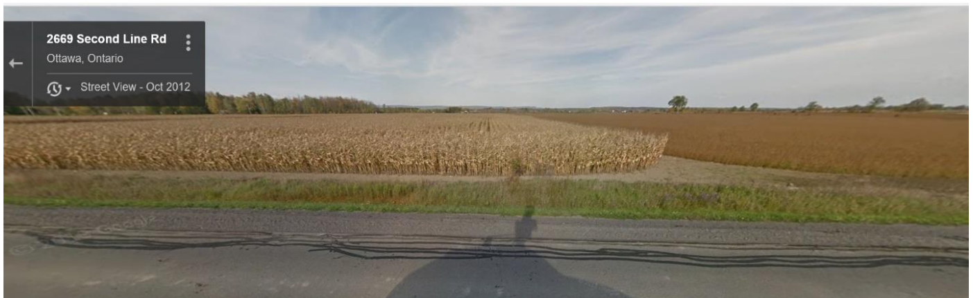
Repair “ribbons” on Second Line Road, Ottawa
